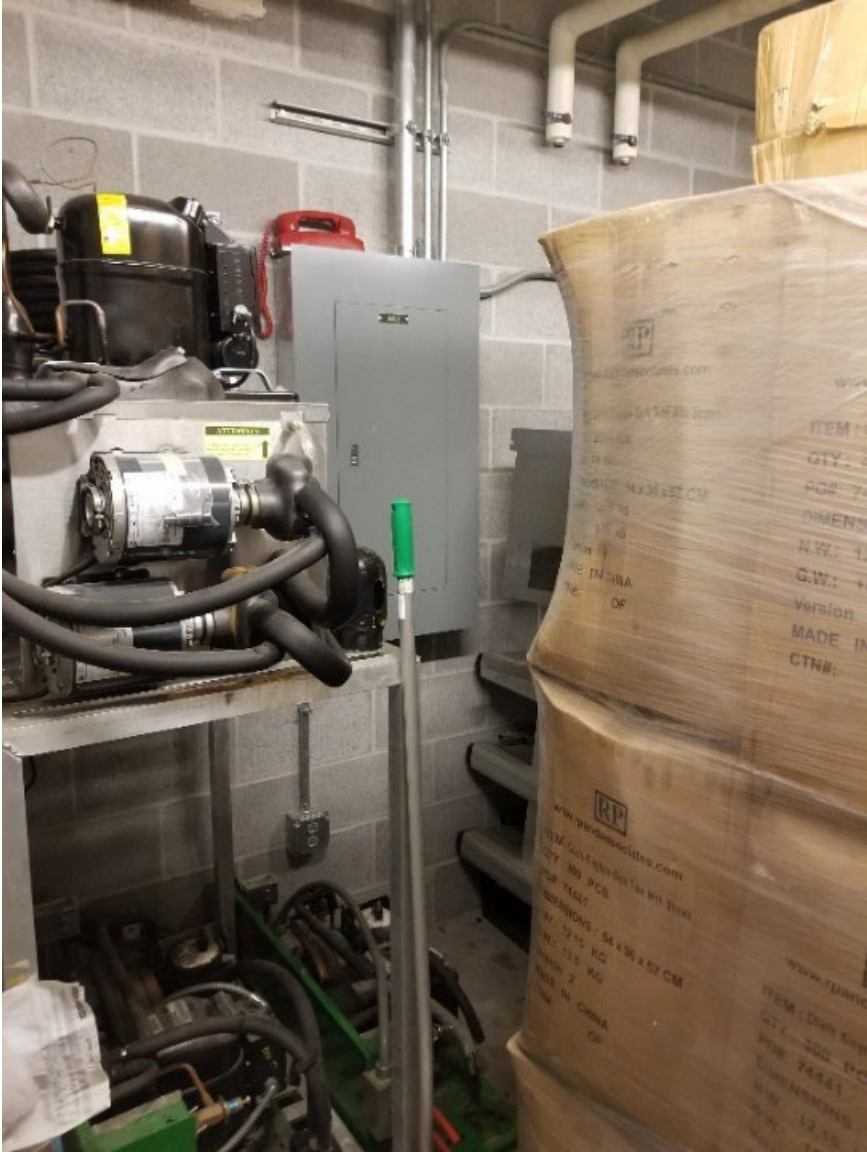
Figure E-2: Inaccessible Panelboard Location: Electrical Room P251
