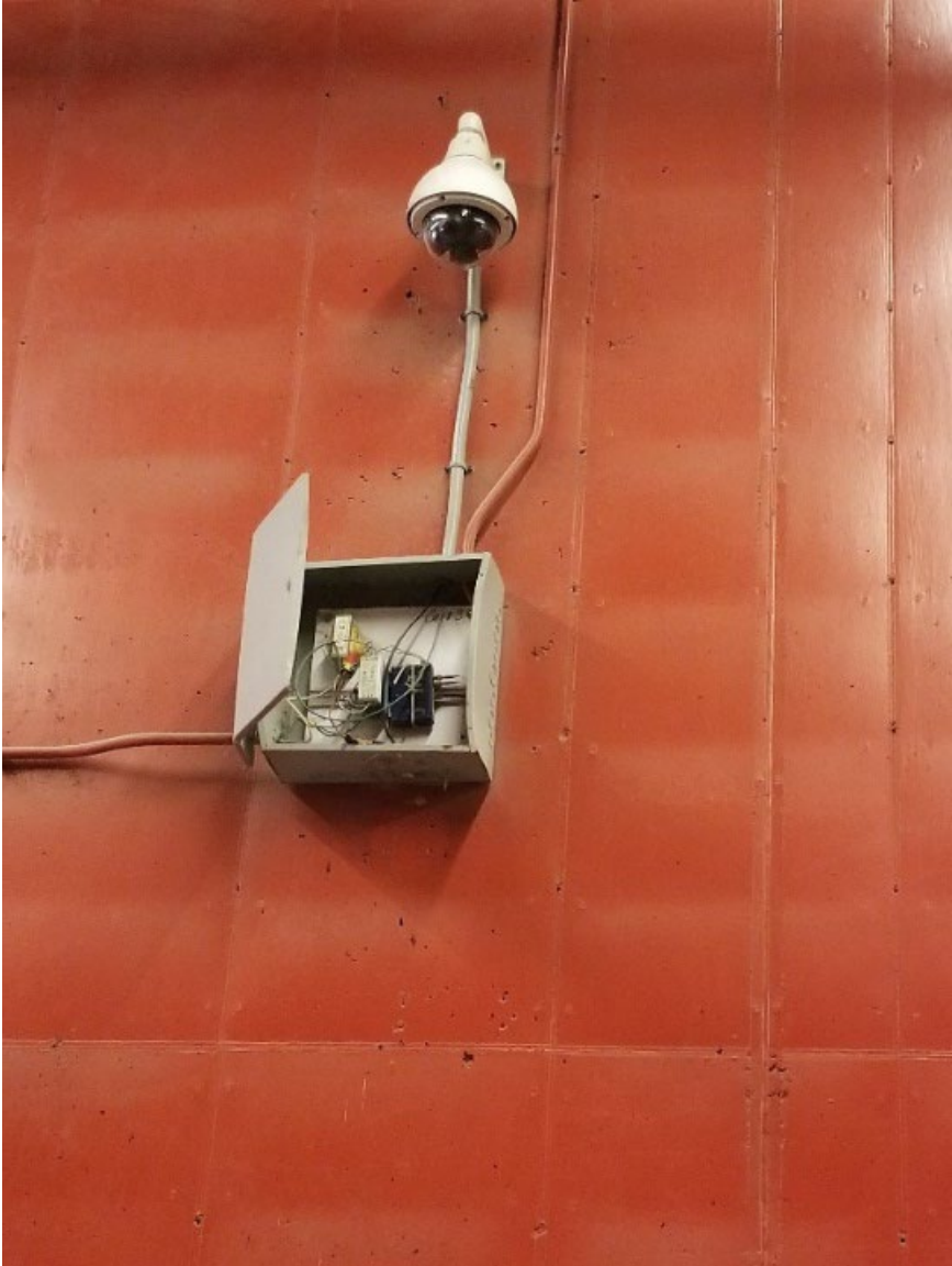
Figure E-4: Exposed Security Enclosure Location: Tunnel 01.55.01
