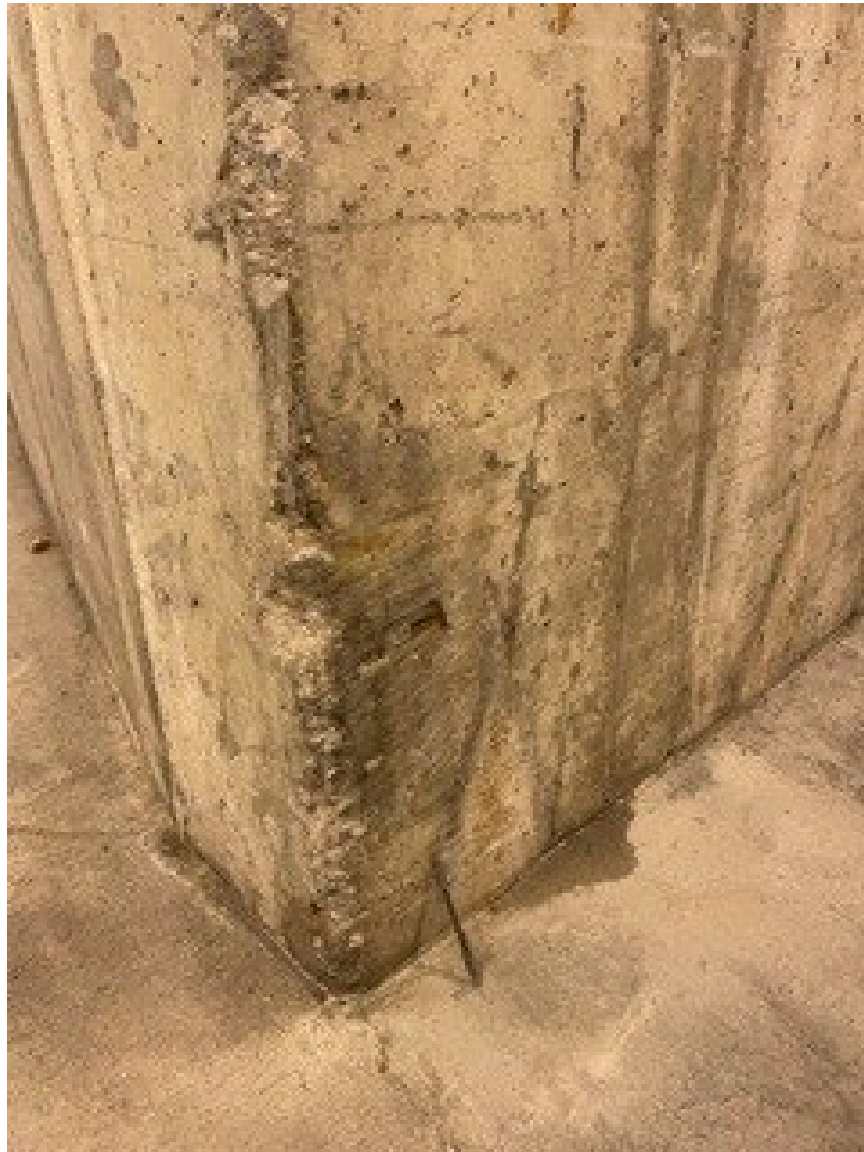
Figure S-1: Concrete Spalling Location: Typical Outdoor Spaces
