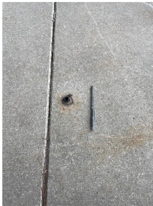
Figure C-5: Tripping Hazard, Exposed Metal Piece Location: All Gates
