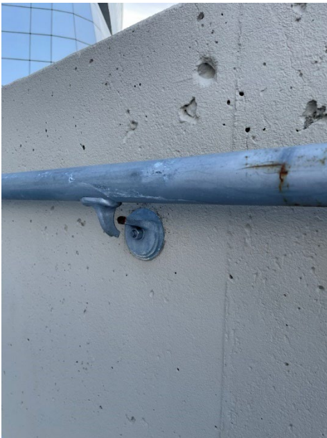
Figure S-4.3: Broken Handrail Support Location: All Helix Ramps
