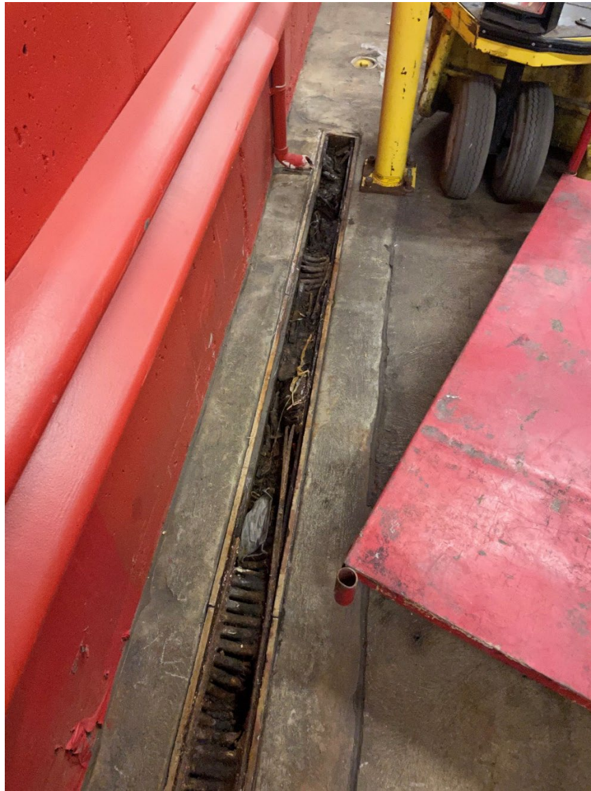
Figure C-12: Rusted, Deteriorated Trench Drain, Full of Trash Location: Chief's Side, Underground Service Corridor
