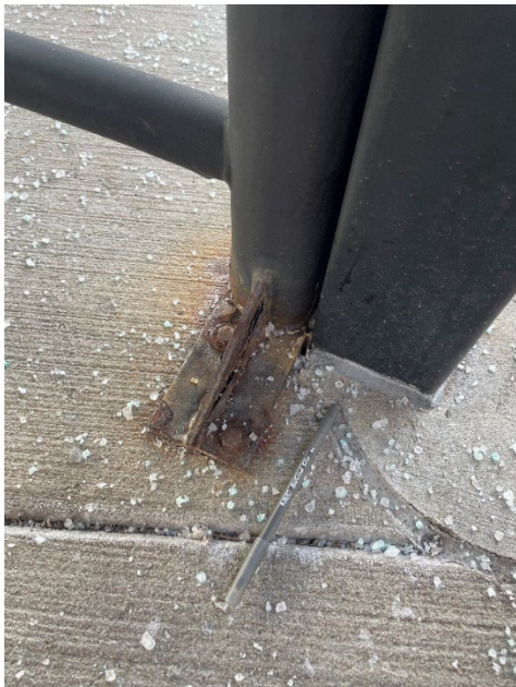
Figure C-2.3: Rusted, Deteriorated Pedestrian Turnstile Location: GEHA Gate
