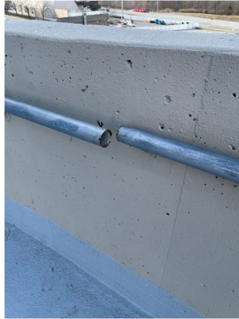
Figure S-4.2: Broken Connection Location: All Helix Ramps
