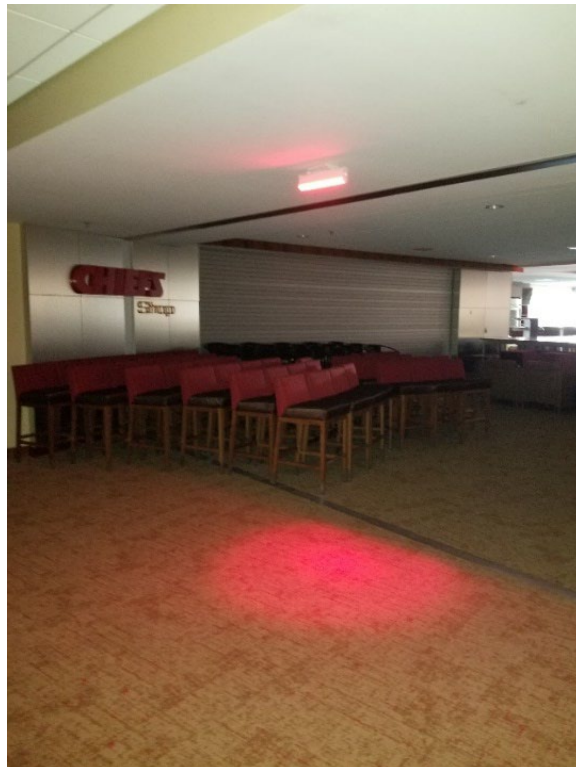
Figure E-1: Exit Sign Missing Location: Outside Suite 240R
