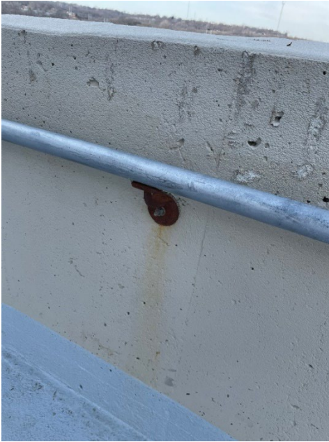
Figure S-4.1: Rusting Handrail Support Location: All Helix Ramps
