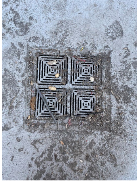
Figure C-9.2: Dirty Floor Drain Grate Location: Upper Concourse
