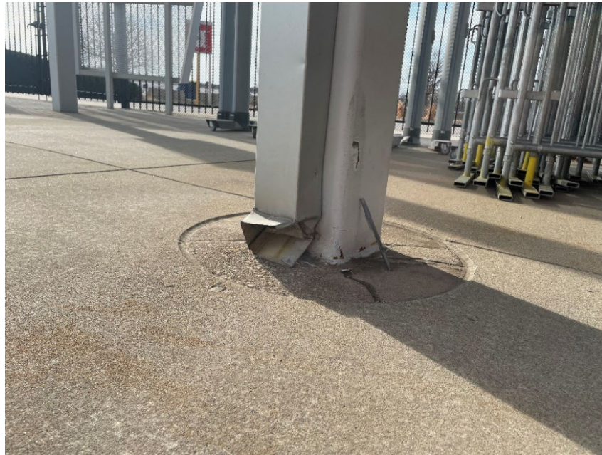
Figure C-4: Dented Rainspout on Canopy Column Location: GEHA Gate
