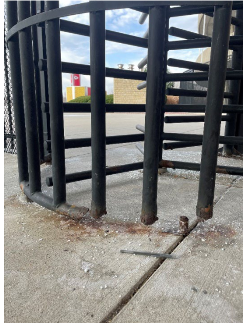
Figure C-2.2: Rusted, Deteriorated Pedestrian Turnstile Location: GEHA Gate
