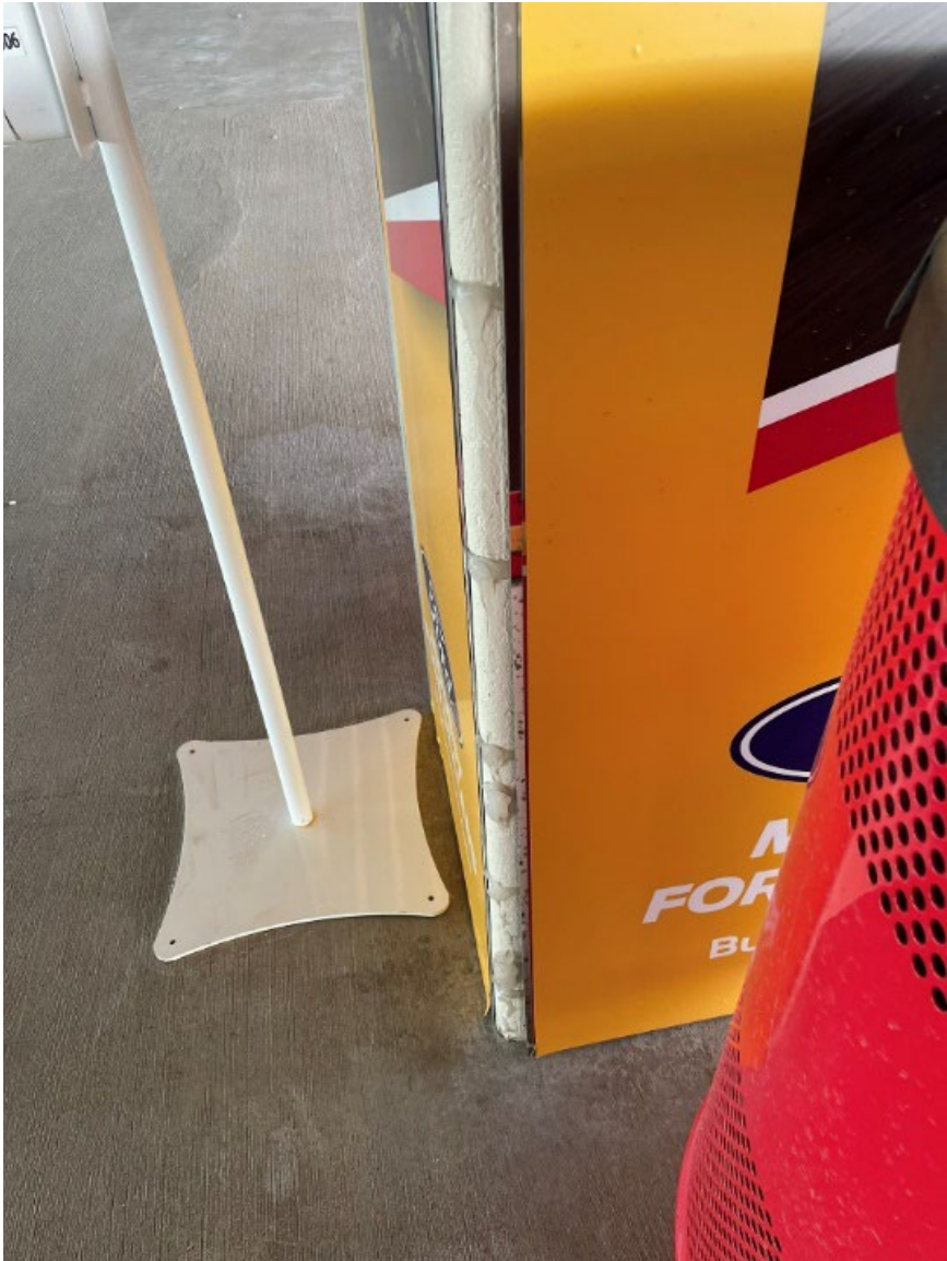
Figure AME-2: Missing Corner Guard Location: Level 8 - Outdoor
