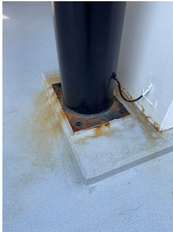
Figure S-2: Rust & Corrosion of Column Location: Level 6 Upper Concourse
