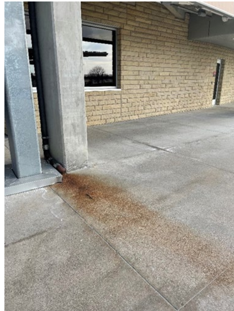
Figure C-1.2: Wider View of Figure C-1 Concrete Discoloration Location: Outside of Security, Between Gate C and T-Mobile Gate
