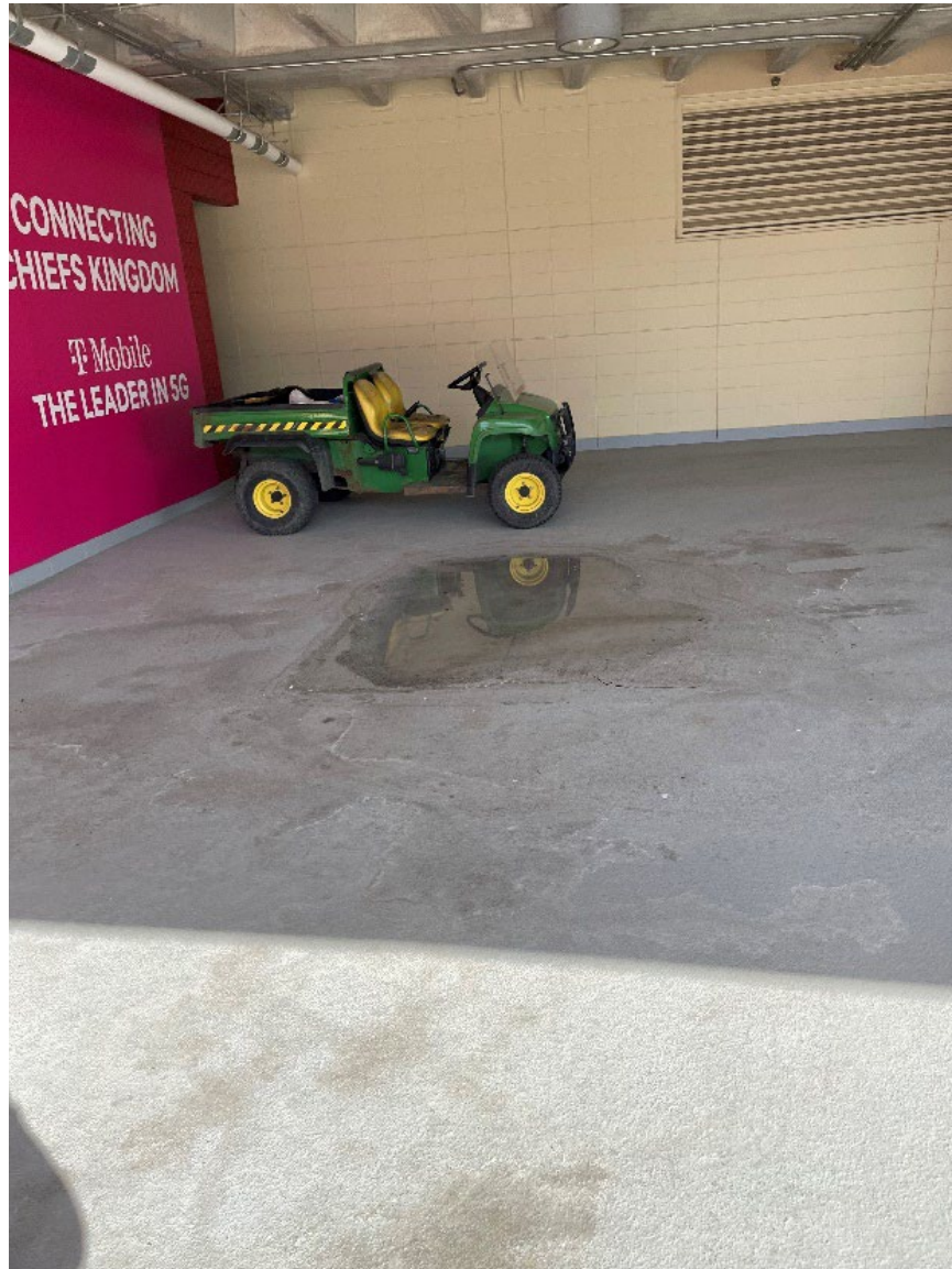
Figure C-11: Upper Concourse Holding Water Location: Top Level, T-Mobile Helix Ramp
