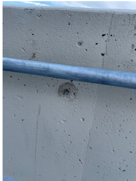
Figure S-4.4: Missing Handrail Support Location: All Helix Ramps
