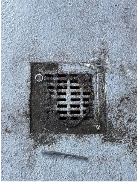
Figure C-9.1: Dirty Floor Drain Grate Location: Upper Concourse
