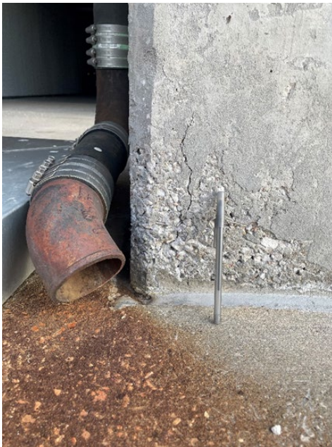
Figure C-1.1: Concrete Discoloration and Eroded Concrete Column Location: Outside of Security, Between Gate C & T-Mobile Gate
