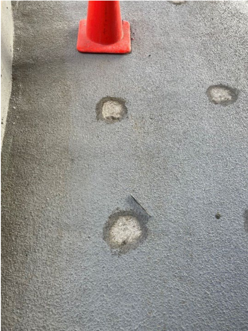
Figure C-6: Epoxy Testing Areas, Tripping Hazard Location: All Helix Ramps
