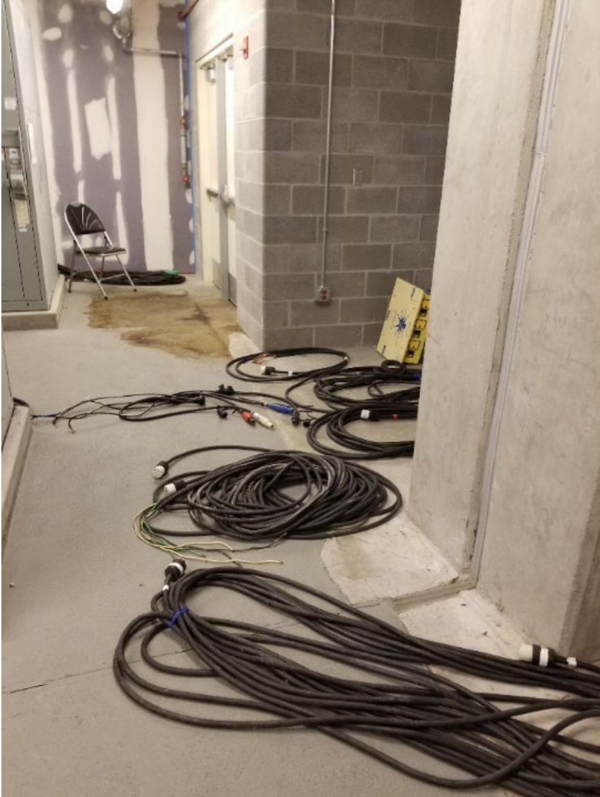
Figure E-3: Cords on the Floor Location: Electrical Room 03.42.02
